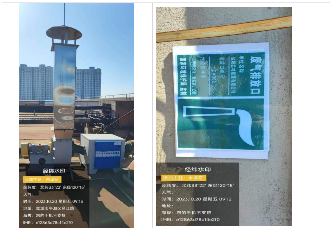
DA002 排气筒及标识
